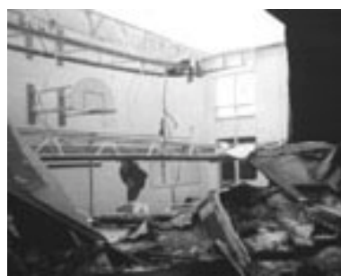
Roof fails from wet snow overload at Claypit Elementary School in Wayland, MA, 2003.
